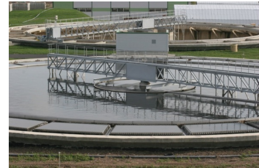
Restoring the ecological health of the Baltic Sea. Southwest Wastewater Treatment Plant in St. Petersburg, Russia.
