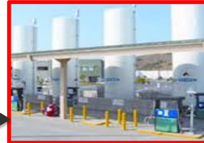
LNG/CNG Filling station
